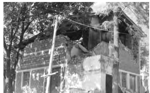
Figure 6.1 : A Damaged Building Due to an Earthquake
